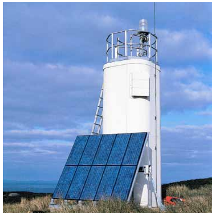
Prefabricated glass reinforced plastic (GRP) cabinet with solar panels installed at North East Island, one of the Kent Group in Bass Strait in 1987. Similar ones have been installed since the mid-1960s in many other locations, in some cases replacing existing light-
